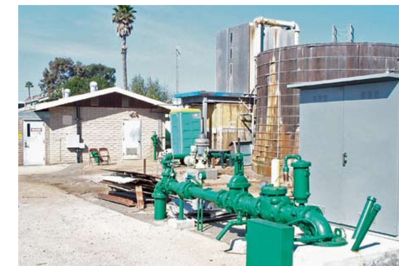
A GROUNDWATER PRODUCTION SITE INCLUDES A WELL AND TREATMENT AND STORAGE FACILITIES
