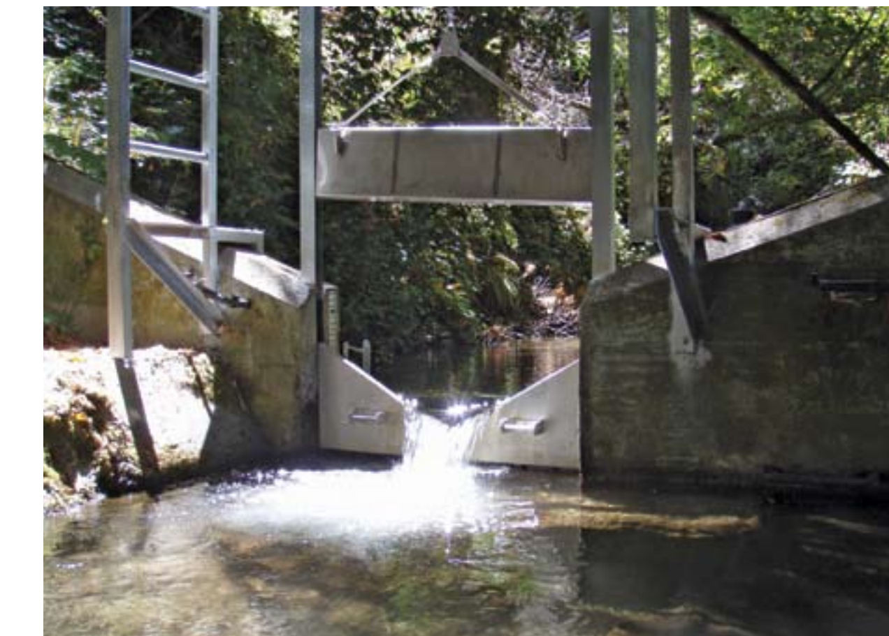
A STREAM DIVERSION TAKES DOMESTIC WATER SUPPLY DIRECTLY FROM A CREEK OR RIVER
