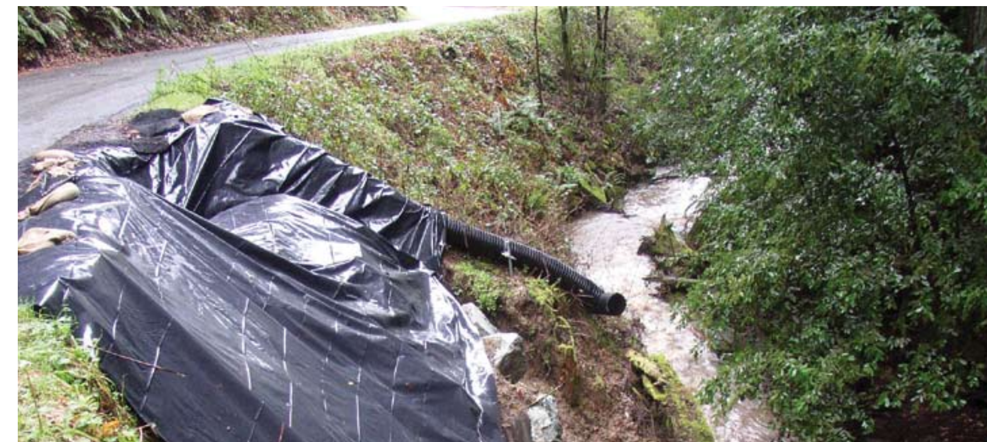
THIS ROAD SLIP OUT DELIVERS SEDIMENTS DIRECTLY TO THE STREAM
