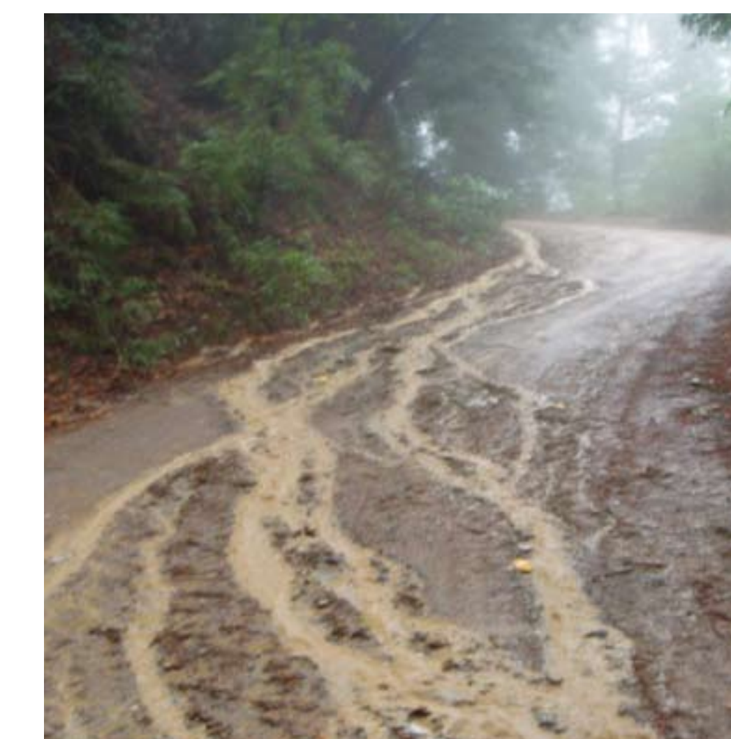
PROPER DRAINAGE ON DIRT ROADS CAN PREVENT EROSION AND REDUCE MAINTENANCE COSTS
